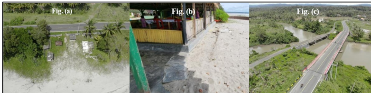
Figure 5. Abrasion impacts (a) Villa; (b) restaurant; (c) bridges (Source: Research Documentation, 2025)
