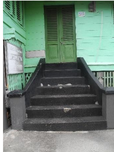
Figure 5. Rumoh Aceh in Materials for the Staircase, which was originally made of wood but is now made of concrete
