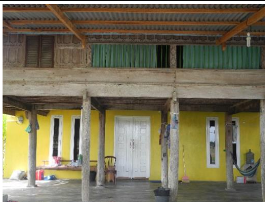
Figure 3. Bottom View of Rumoh Aceh Section that has been Modified with a Concrete Structure
