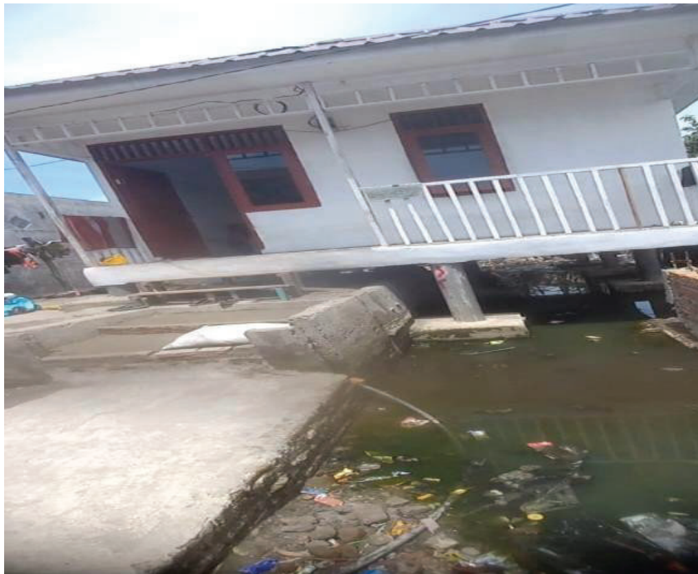
Figure 6. Waste Accumulation in Residential Drainage Channel
