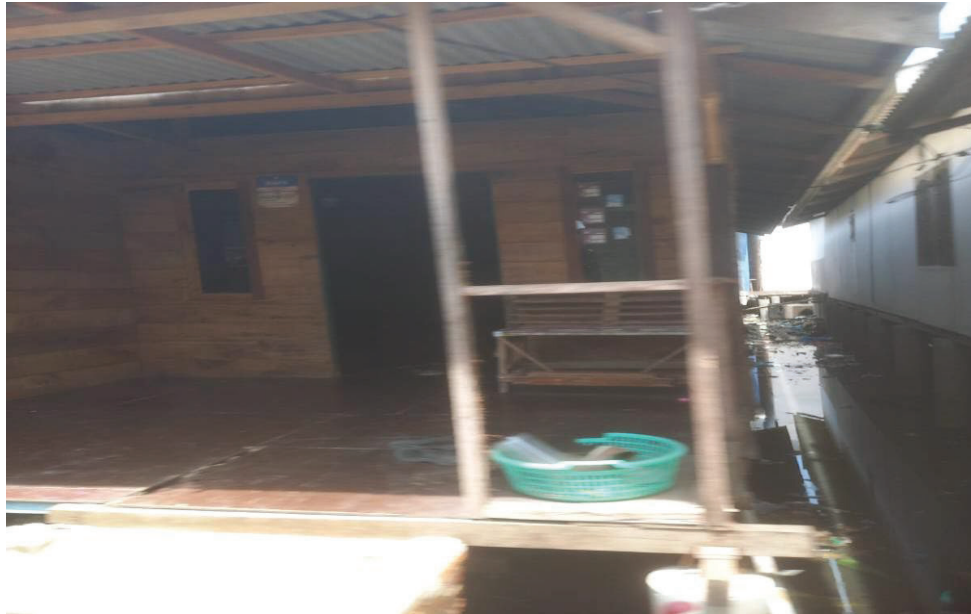
Figure 7. Standing Water Observed Between Residential Buildings Author Documentation, 2026
