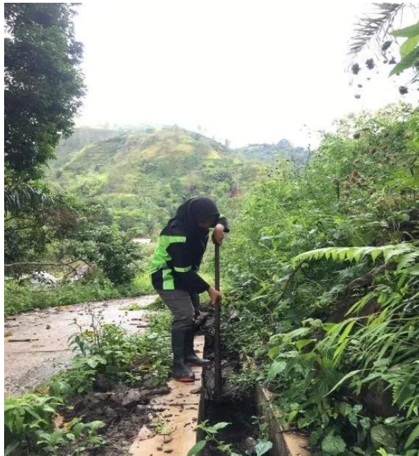
Fig. 2. Cleaning the road to the community home in the village Height, Dusun 11
